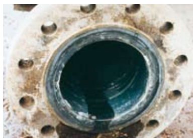
Removal of solidified bauxite from pipes upper: prior to cleaning lower: after cleaning
