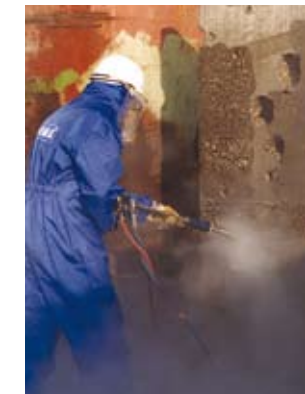
Partial concrete removal and exposing of reinforcements with hand-held water jet tools
